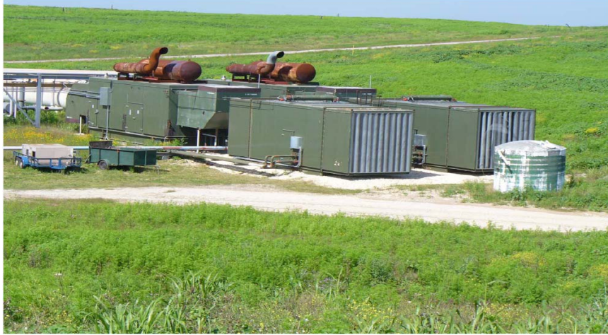
Gas-fired peaking units installed in Texas
