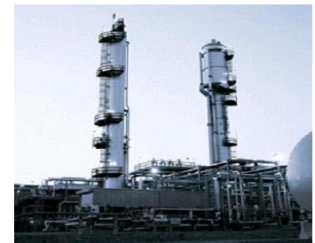
Joffre ethane extraction plant
