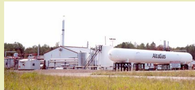
Sylvan Lake gas plant
