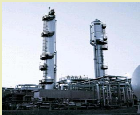
Joffre ethane extraction plant
