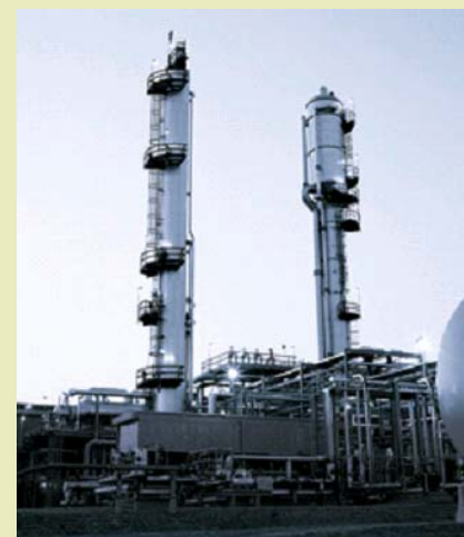
Joffre Ethane Extraction Plant
