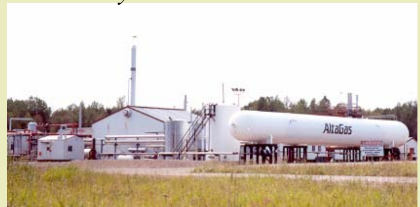
Sylvan Lake Gas Plant
