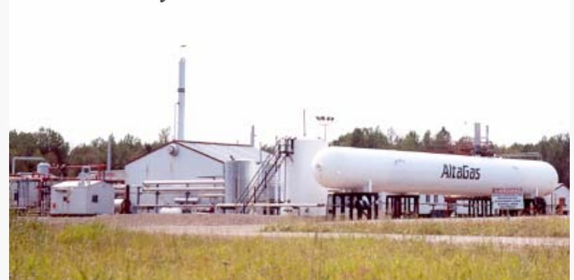
Sylvan Lake Gas Plant
