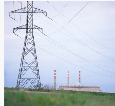
Sundance B Power Plant
