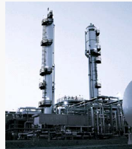
Joffre Ethane Extraction Plant
