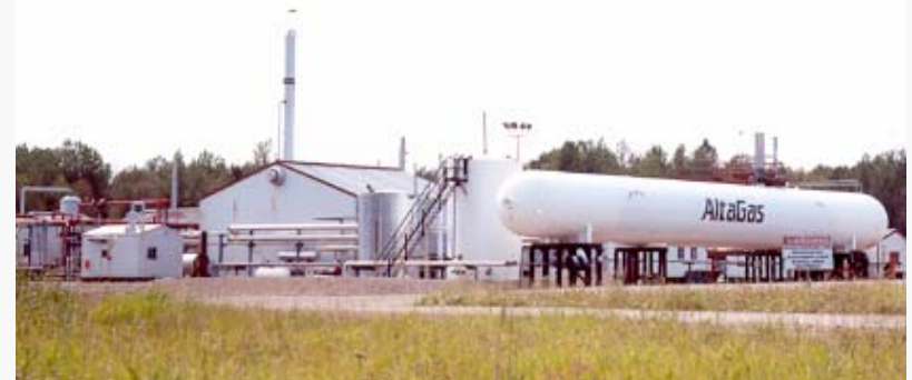
Sylvan Lake Gas Plant
